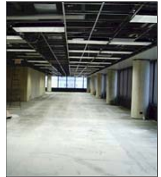
Terra's Centre's sixth floor in the middle of the demolition process. Within the next several months, this floor and half of the seventh floor will undergo further transformation.
